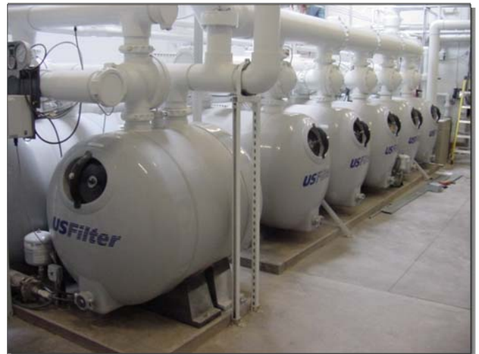
Mechanical Filtration Systems
